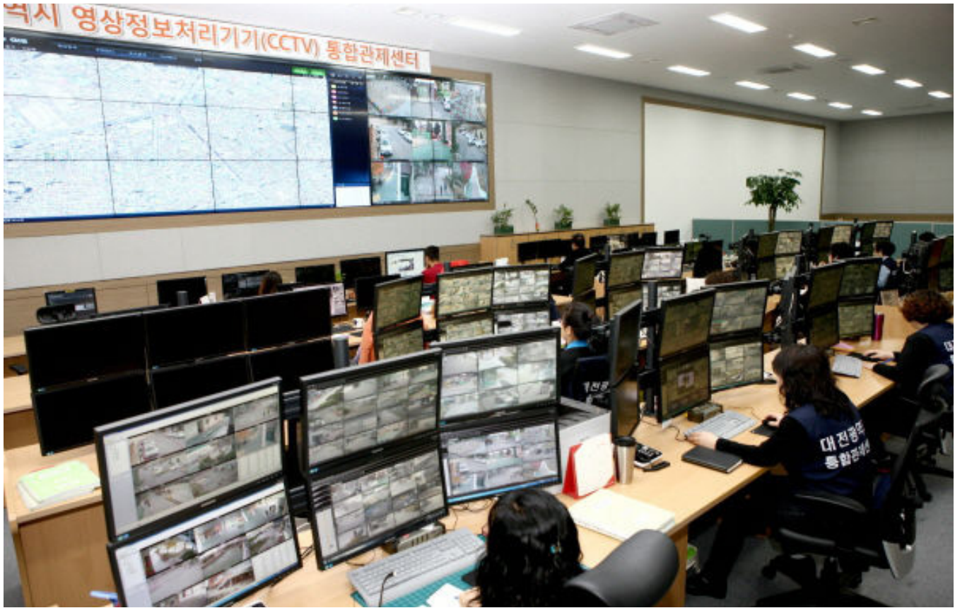
FIGURE 2. THE CCTV CONTROL CENTER IN THE DAEJEON SMART CITY OPERATION CENTER
